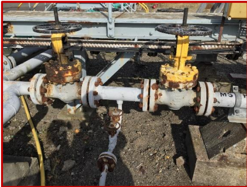
Existing Defective Valves & Bobbin
